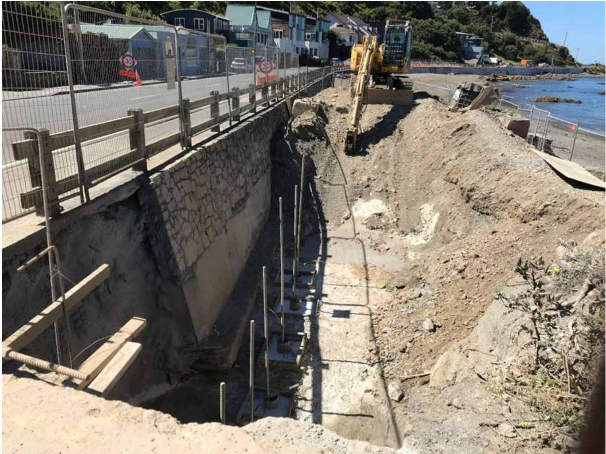
Figure 2.7. Replacement of the circa 1930's mortared brick seawall on the eastern side of Ōwhiro Bay.
