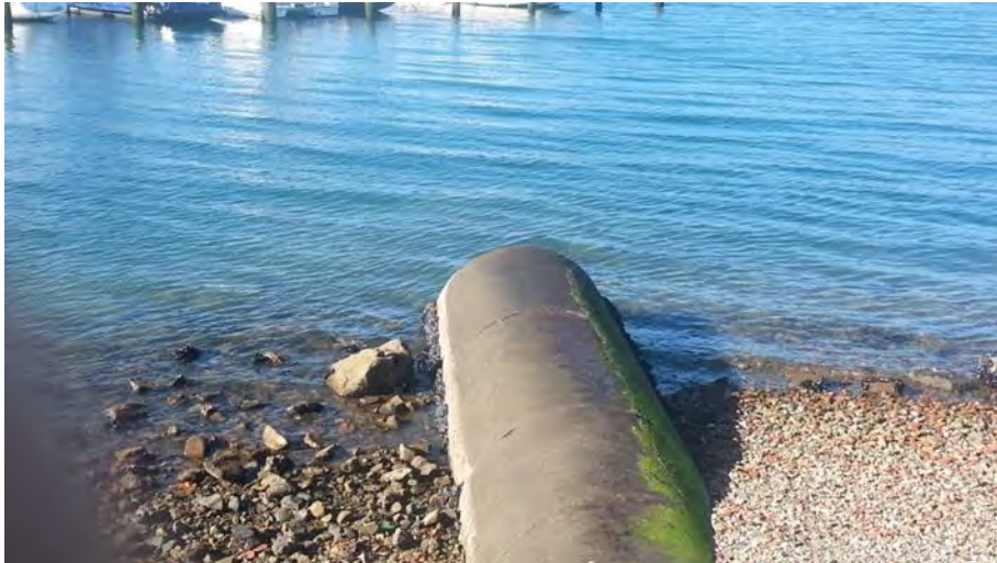
Figure 22: Stormwater outfall Kilbirnie
