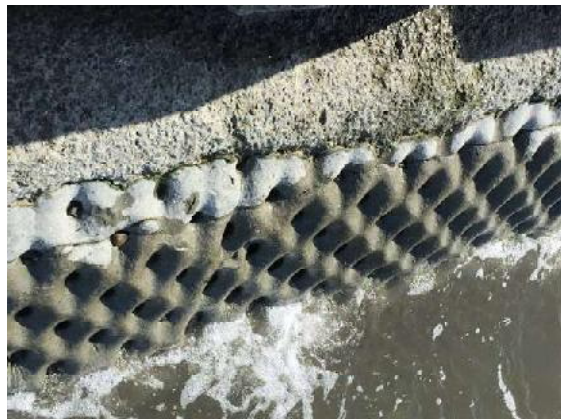
Photo 38: Seawall face with no marine invertebrate colonisation.
