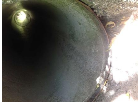
Photo 12: Rain flow discharging pipe.
